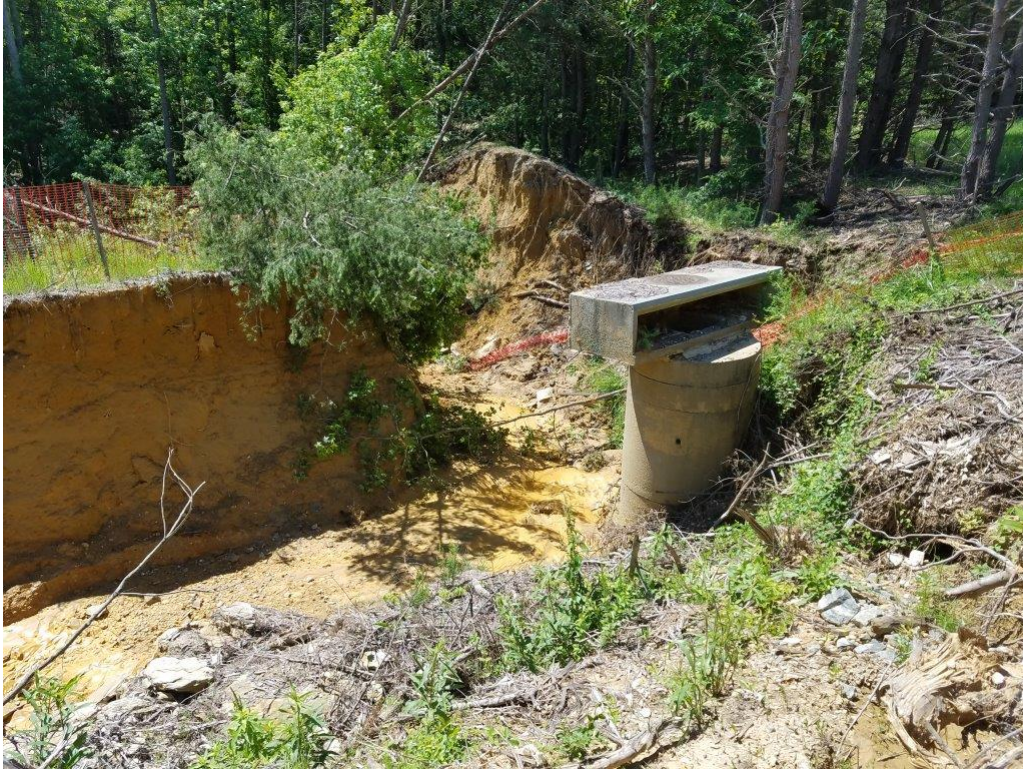
Erosion Issue on TMP 38-14G
