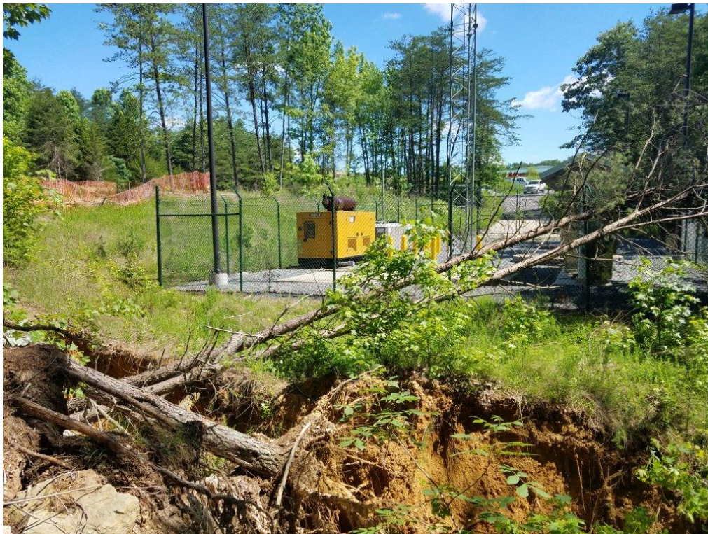
North Stafford Industrial Park Sewage Pump Station
